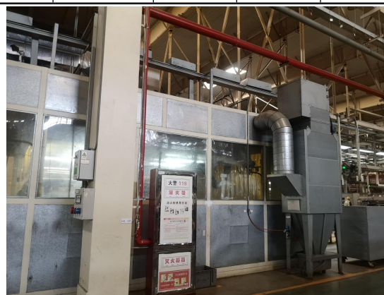
焊接烟尘滤筒除尘 2
