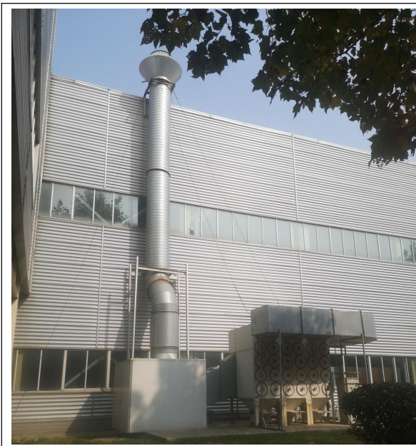
焊接烟尘滤筒除尘 3
