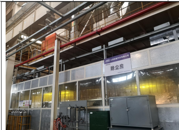
焊接烟尘滤筒除尘 1
